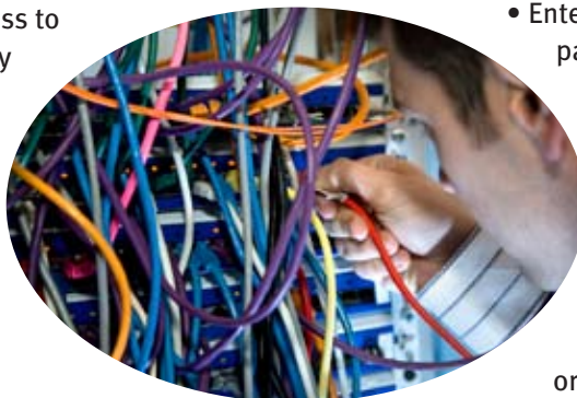
Avoid IT wiring headaches with a wireless solution
